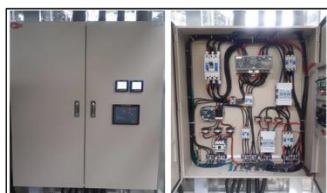
Switches of Interconnected System
